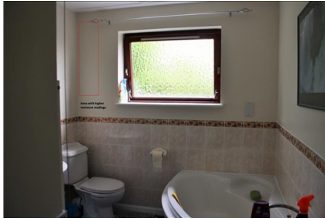
Main bathroom showing area with damp
