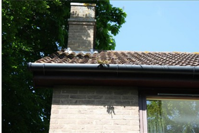
Rear Roof, leaves on roof and in gutter
