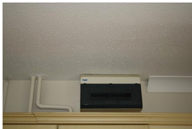
Consumer unit, above kitchen cupboard
