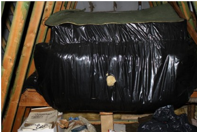
Cold water tank in loft space
