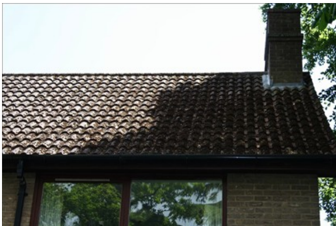
Front roof, some moss and leave covering
