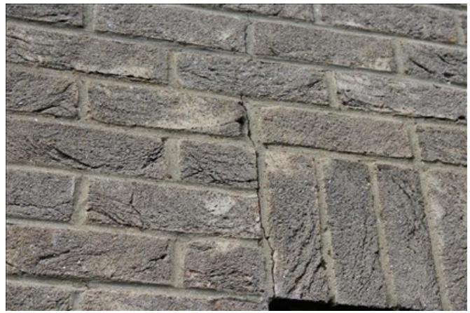
Crack to wall above patio doors
