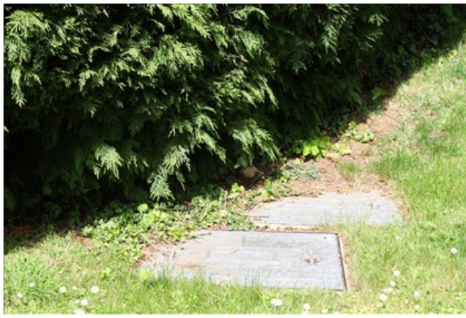
Inspection chambers not opened
