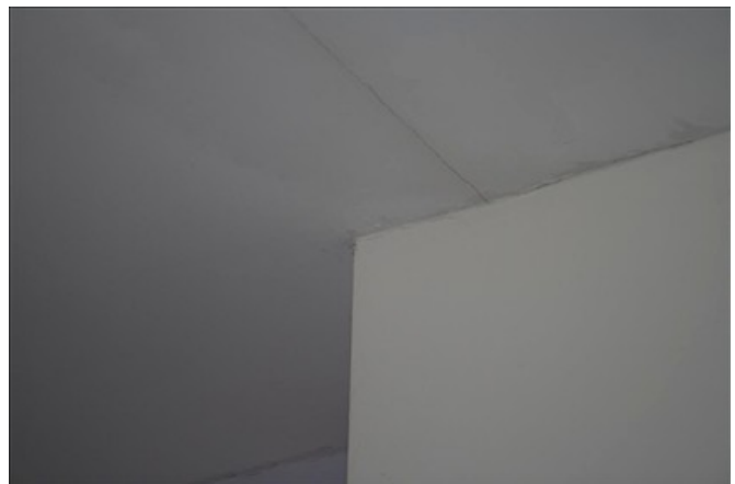
cracking along ceiling plasterboard joints
