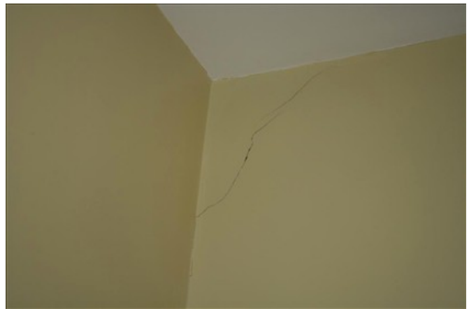
cracking in Dining Room
