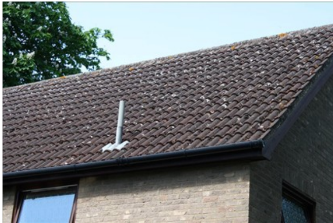
uncapped soil and vent pipe
