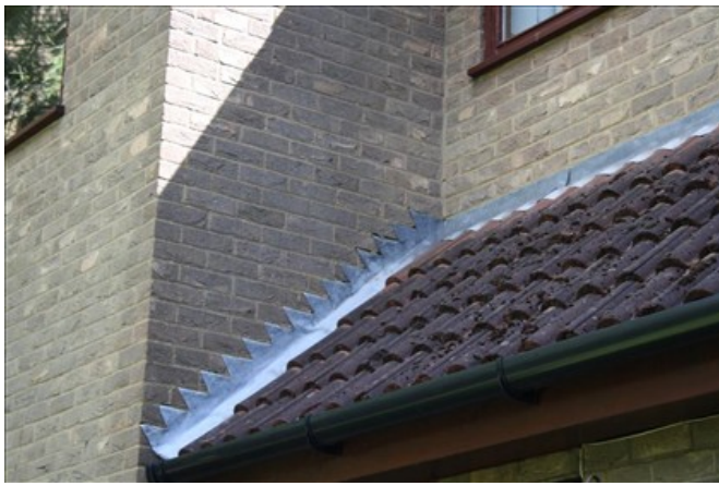
porch roof meets wall - some missing mortar
