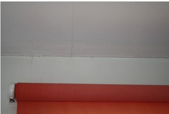
minor cracking where ceiling meets wall
