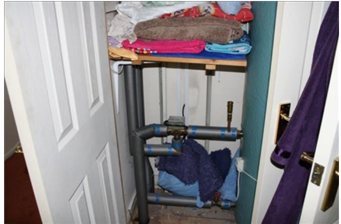
Hot water cylinder and insulated pipes
